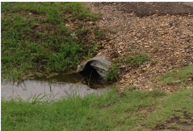
Figure 7A: Damaged Culvert Example
