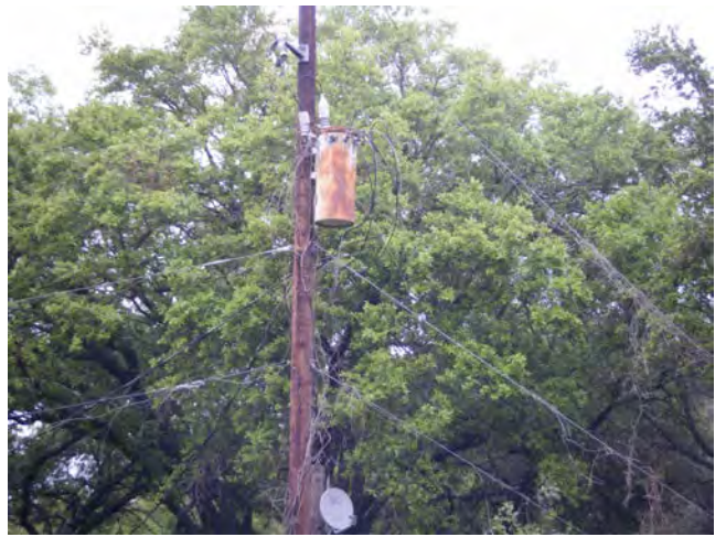
RUSTED TRANSFORMER – NORTH OF SITE WEST OF BUSINESS 59
